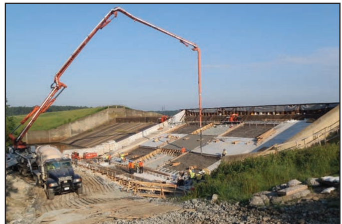
Diascund Creek Reservoir Dam's principal spillway now includes a more robust underdrain system, improved steel reinforcement, and polyvinyl chloride (PVC) waterstops for improved water-tightness.
